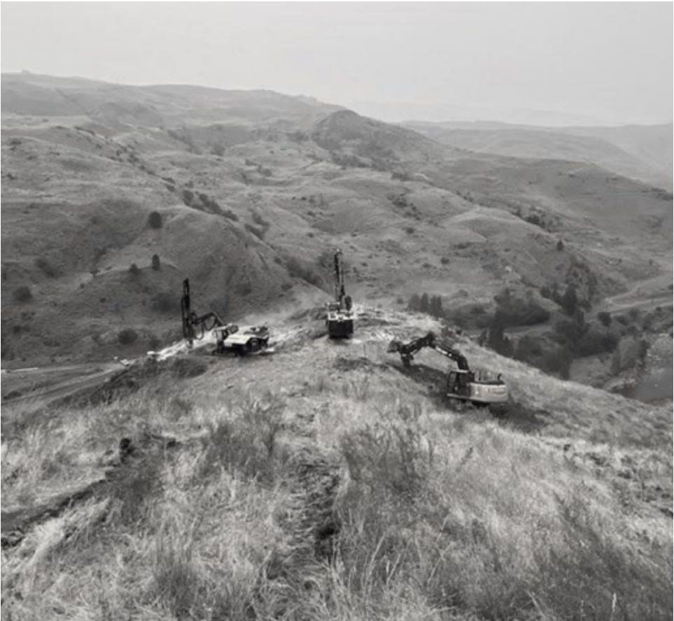
Figure 11. Ryno Works drilling under tough conditions, at 40+C with wildfire smoke filling the horizon. Trim blastholes were drilled at 56 to 60 degrees sub-parallel to the failure surface of the block. Depth of the blastholes were about 30 m.
