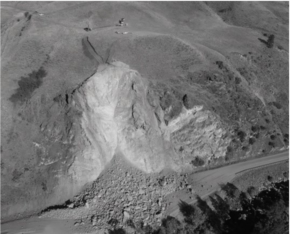
Figure 15. The image displays the muck pile immediately following the dust clearing from the blast. None of the material ended up in the Little Salmon River, a good success.
