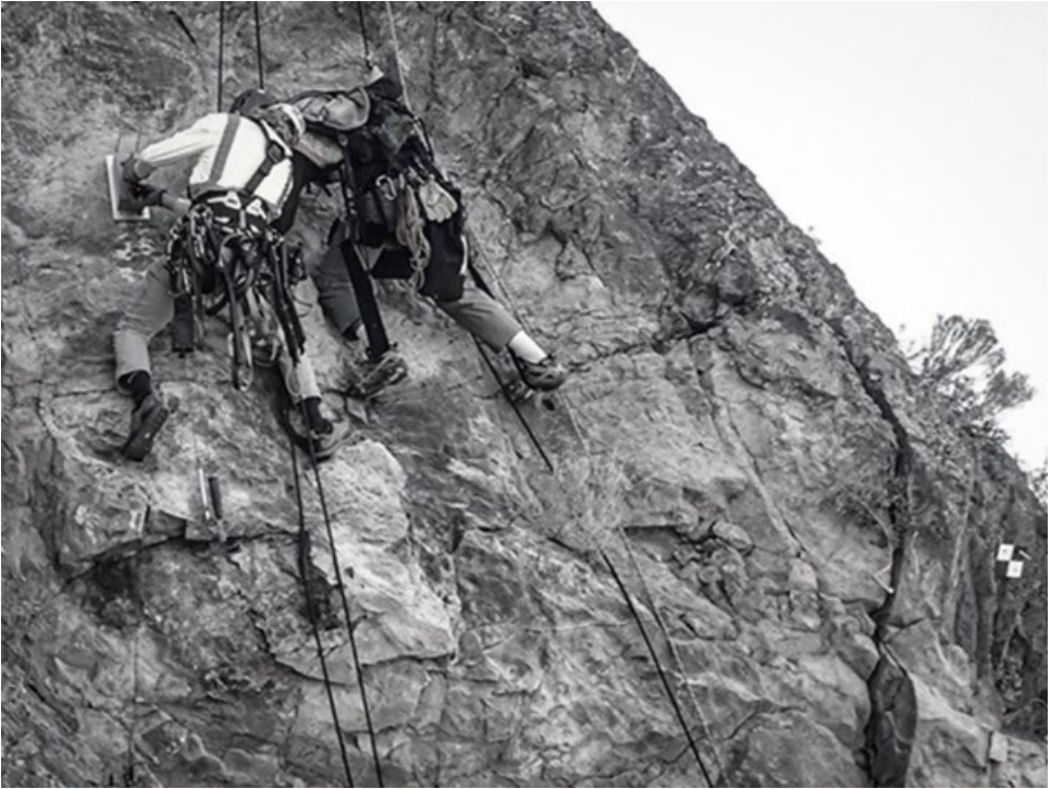
Figure 4. Installation of instrumentation (crack gauges, tilt meters, prisms) total station targets, extensometers.
