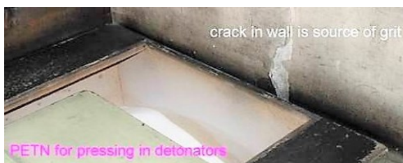
Crack in wall at PETN container is a source of grit (Credit: SAFEX)
